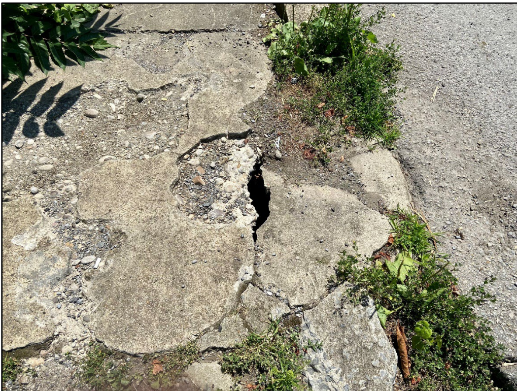
Photo 10: Cracks in North Sidewalk at West Approach. View Southeast.
