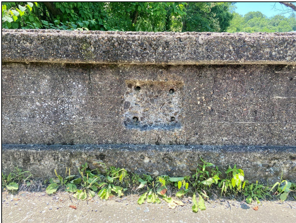
Photo 8: Missing Plaque at West End of South Railing. View Southwest
