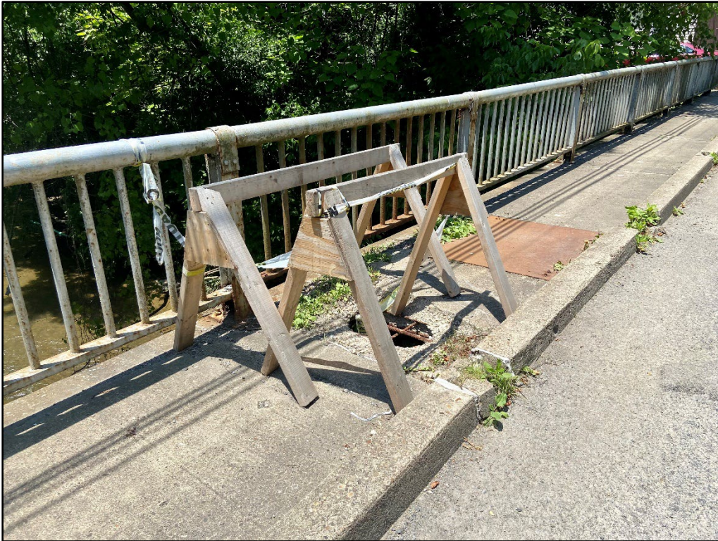
Photo 9: Hole in South Sidewalk Middle of Bridge. View Northwest
